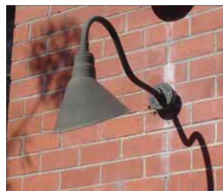
Exterior attached lighting
