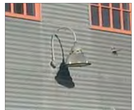
Exterior attached lighting
