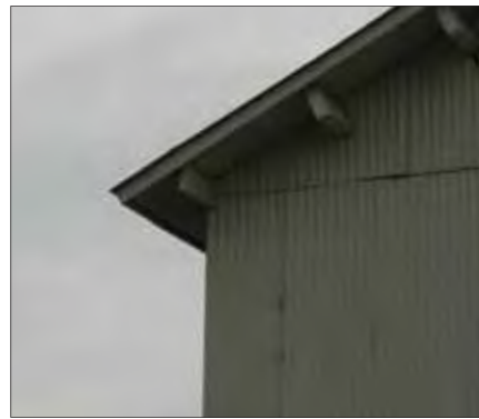
Exposed purlin tails on gable end
