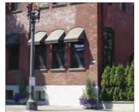
Concrete base is painted a different color than the brick siding
