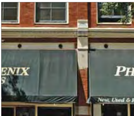
The wall below the base cornice changes material from the brick primary wall and acts as an independent pier
