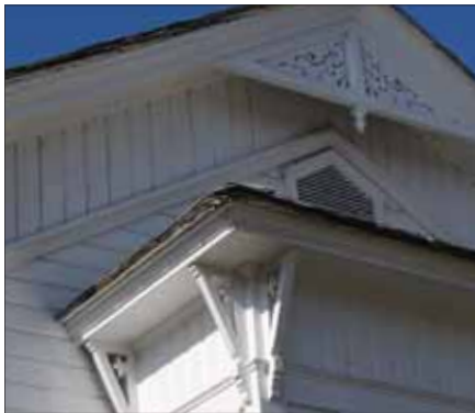
Roof and wall connection on the main body of the house with bracketed bay
