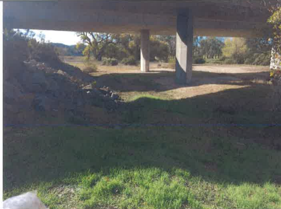
Photo 3. View south from The Ravine to floodplain, left of main channel on the right side of the photo. Timber tramway to be placed between rip-rap and concrete piers. Photo taken November 21, 2016.
