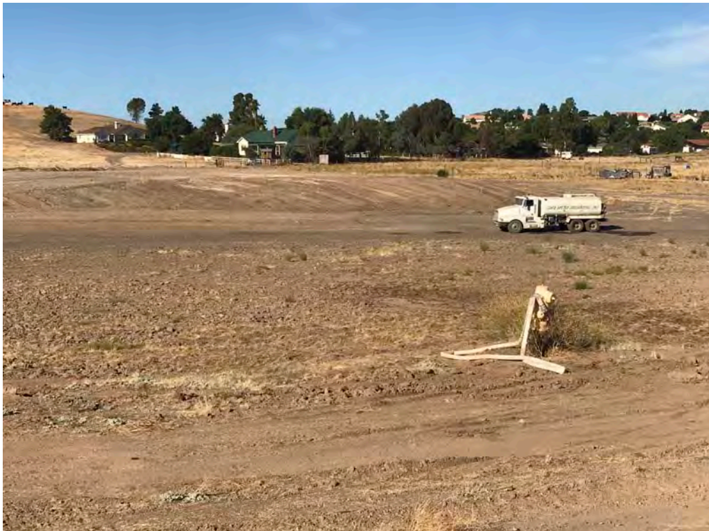
Photo 4. Westerly view of site from eastern property line shows active stockpile management area and residential development to the west in the distance.
