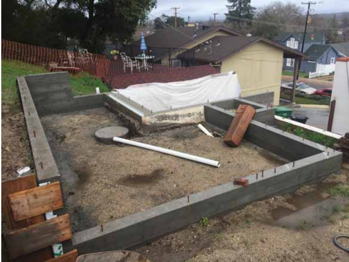
Site Photo 1: View of foundation for the upper level of the guest house addition, looking northeast.
