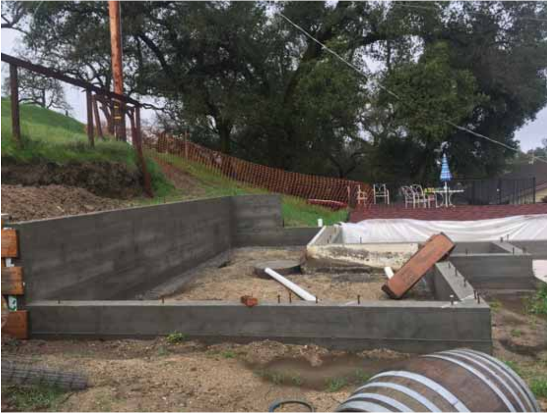
Site Photo 2: View of foundation for the upper level of the guest house addition, looking north.
