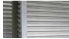
SIDING: 1 1/2" DEEP ALUMINUM WALL PANEL (MATRIX MX1.0 24 GA.) MFR: MORIN. COLOR: GALVALUME TO MATCH EXISTING
