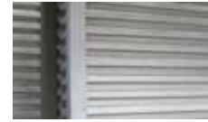
SIDING: 1 1/2" DEEP ALUMINUM WALL PANEL (MATRIX MX1.0 24 GA.) MFR: MORIN. COLOR: GALVALUME TO MATCH EXISTING
