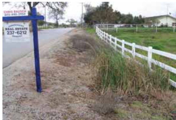
12. A small wetland has formed at the outlet of a culvert draining nuisance water from the adjacent residential development. Photo 2006.
