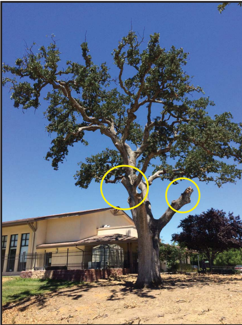
Photo 1- View of tree from southeast. Scaffold failures indicated by yellow circles.
