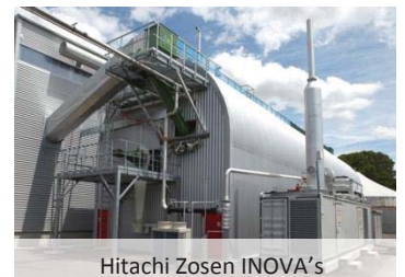
Hitachi Zosen INOVA's Anaerobic Digestion Plant
