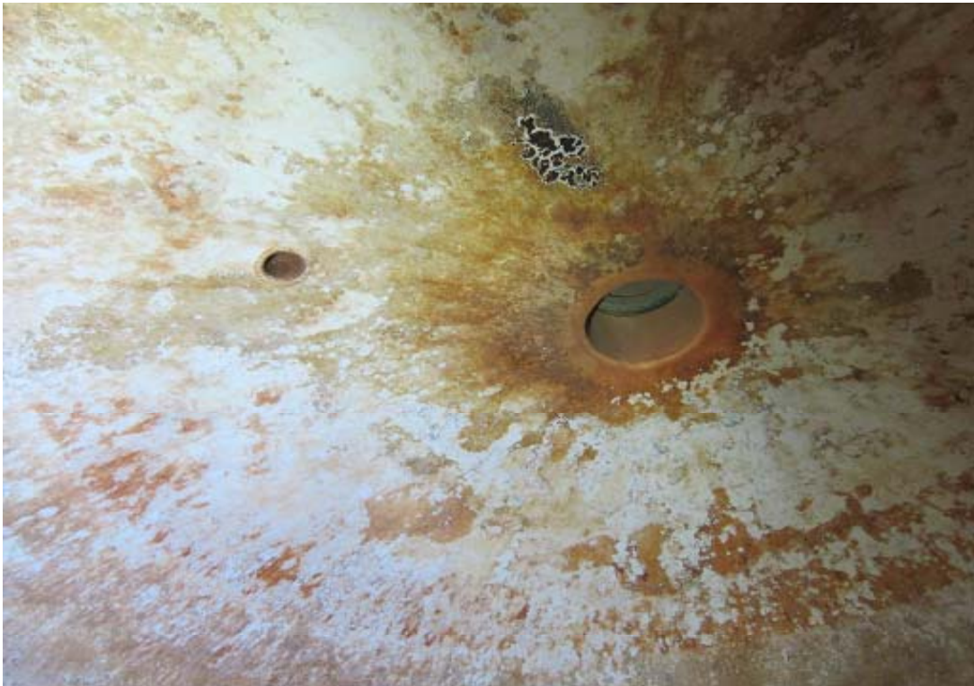
Vessel top head with nozzles with staining and scattered general corrosion. Interior view (existing condition, 4/11/17).
