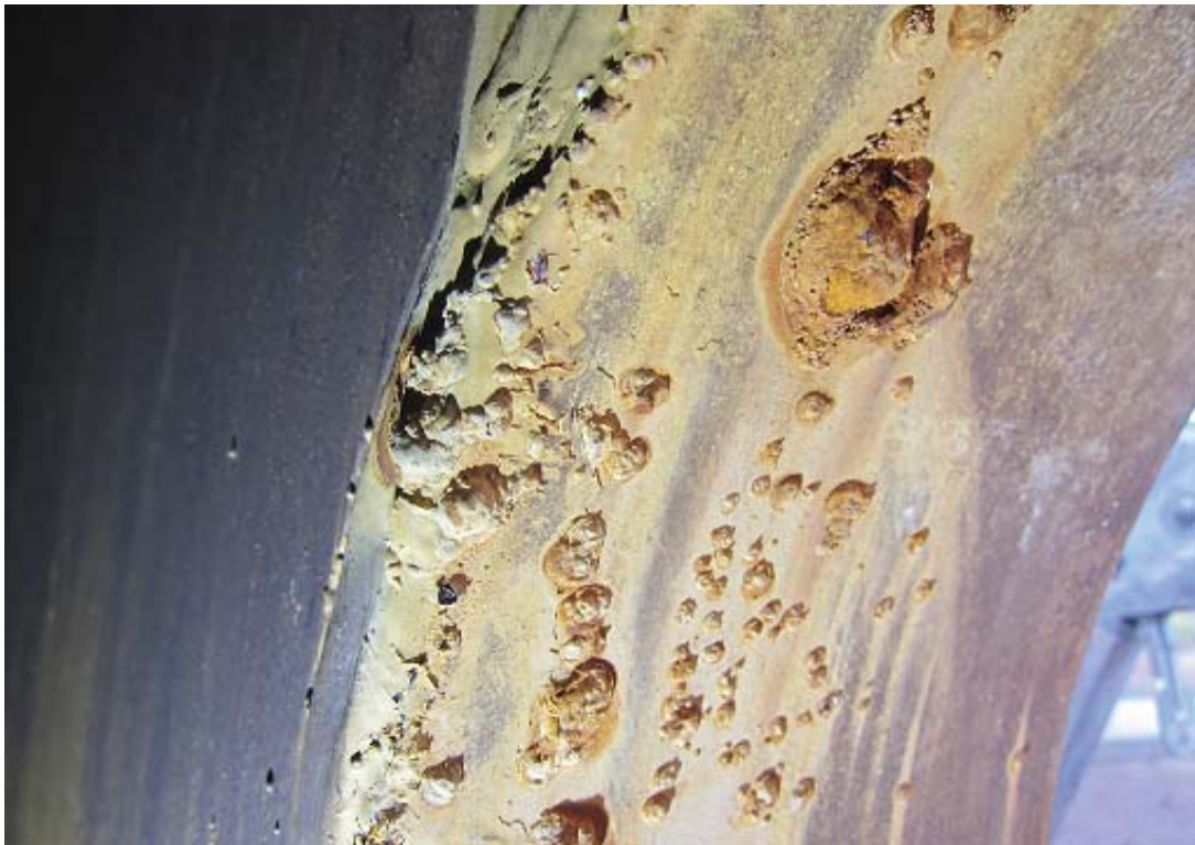
Nodules from localized corrosion on the interior at the manway neck (existing condition, 4/11/17).
