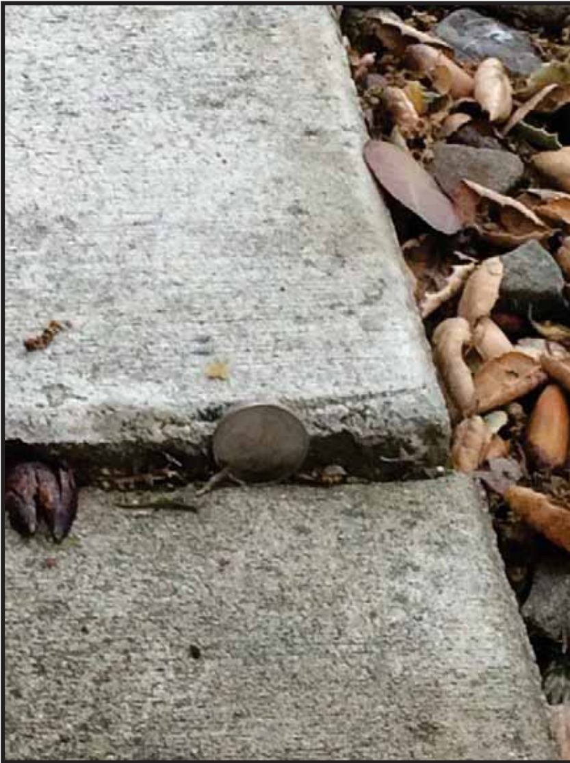
Photo 3- Close -up of sidewalk uplifting next to Tree 1, approximately \frac{3}{4} ".
