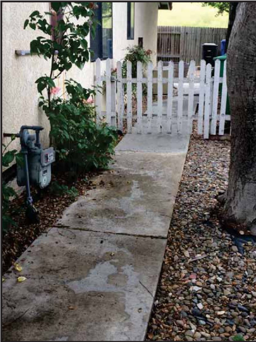
Photo 2- View of Tree 1 roots uplifting sidewalk adjacent to gas meter.
