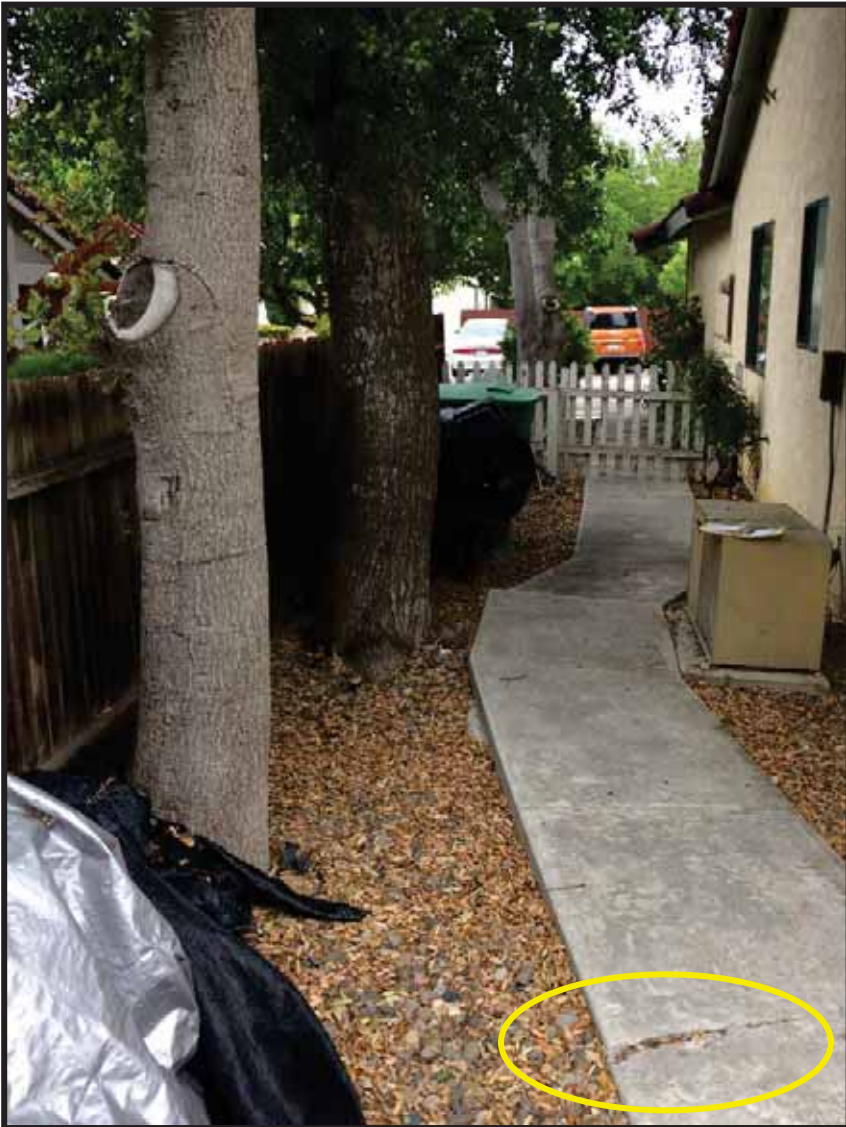
Photo 6- View of sidewalk uplifting next to Tree 3, indicated by yellow circle. Uplift is approximately \frac{3}{4} ".
