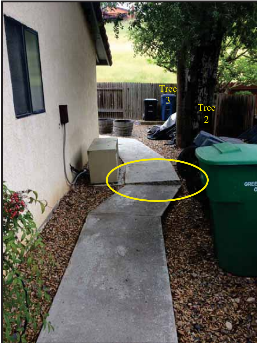
Photo 4- View of sidewalk uplifting next to Tree 2, indicated by yellow circle.
