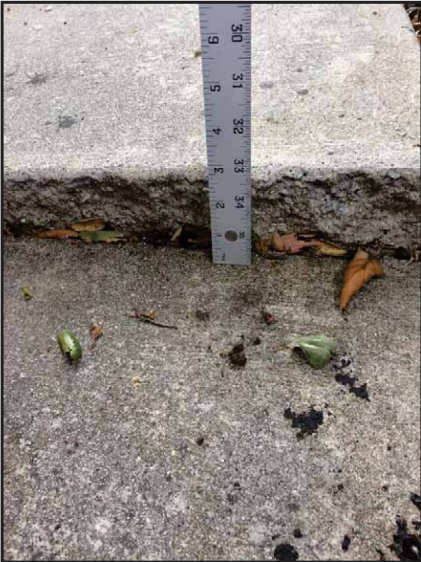
Photo 5- Close- up of sidewalk uplift next to Tree 2, approximately 3".
