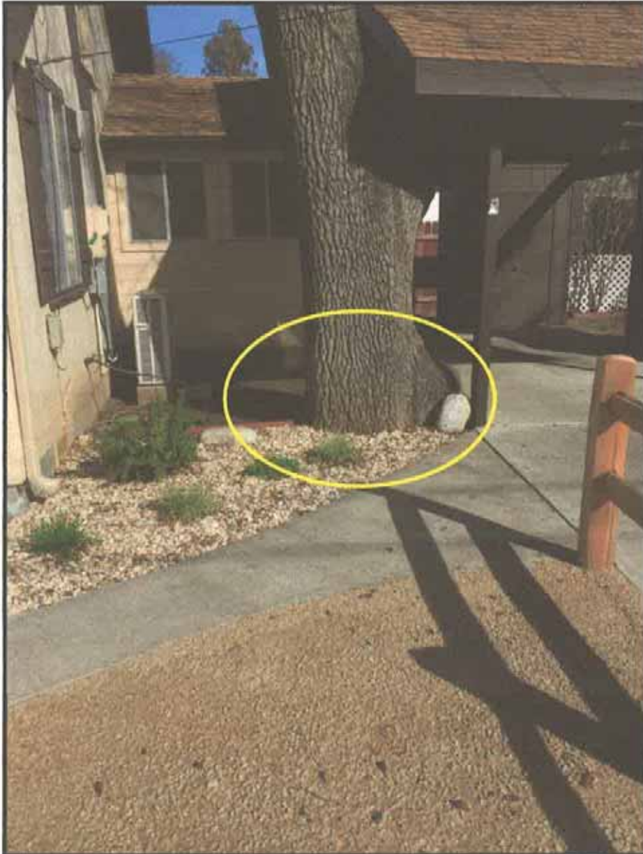
Photo3- Close-up of grade buried root crown and restricted root space.
