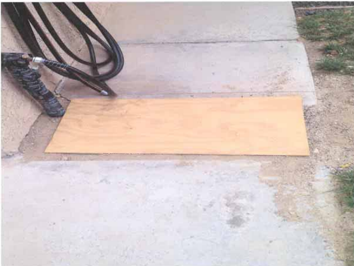
Area where the roots broke the water line
