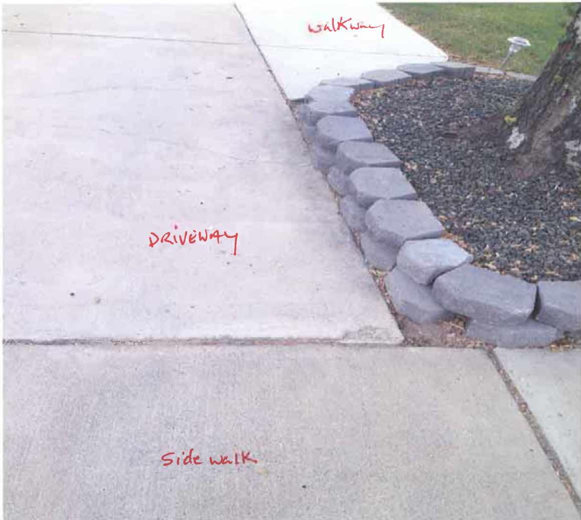
Concrete that was replaced at the top and the crack in the old concrete
