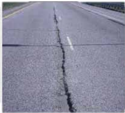
Transverse or Longitudinal Cracking
