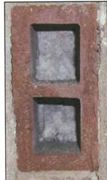
Figure 8: Brick in Cross Section (July 2009)
